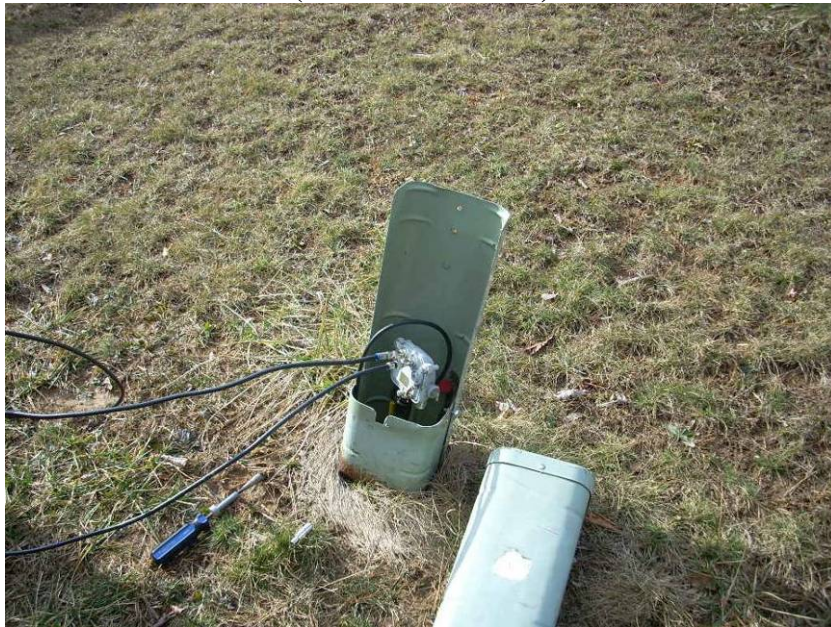
Figure 4: Underground Plant EOL Not Grounded (213 Lincoln Lane)
