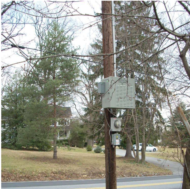
Figure 5: Complaint Aerial Standby Power Supply (Blanker Road and SR 32)
