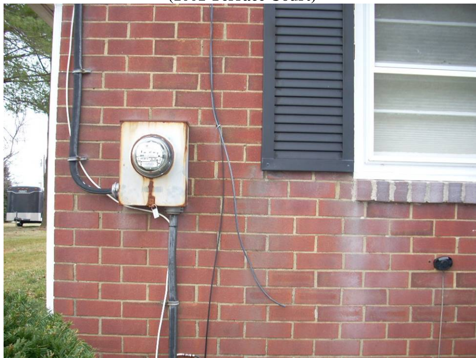
Figure 3: Disconnected Drop Not Grounded (1001 Terrace Court)
