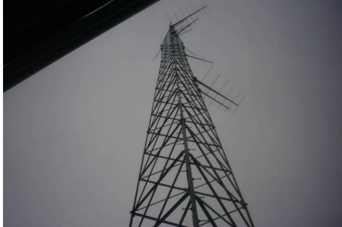
Self Supporting Tower
